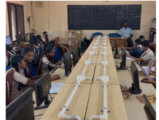
Powering education through solar
